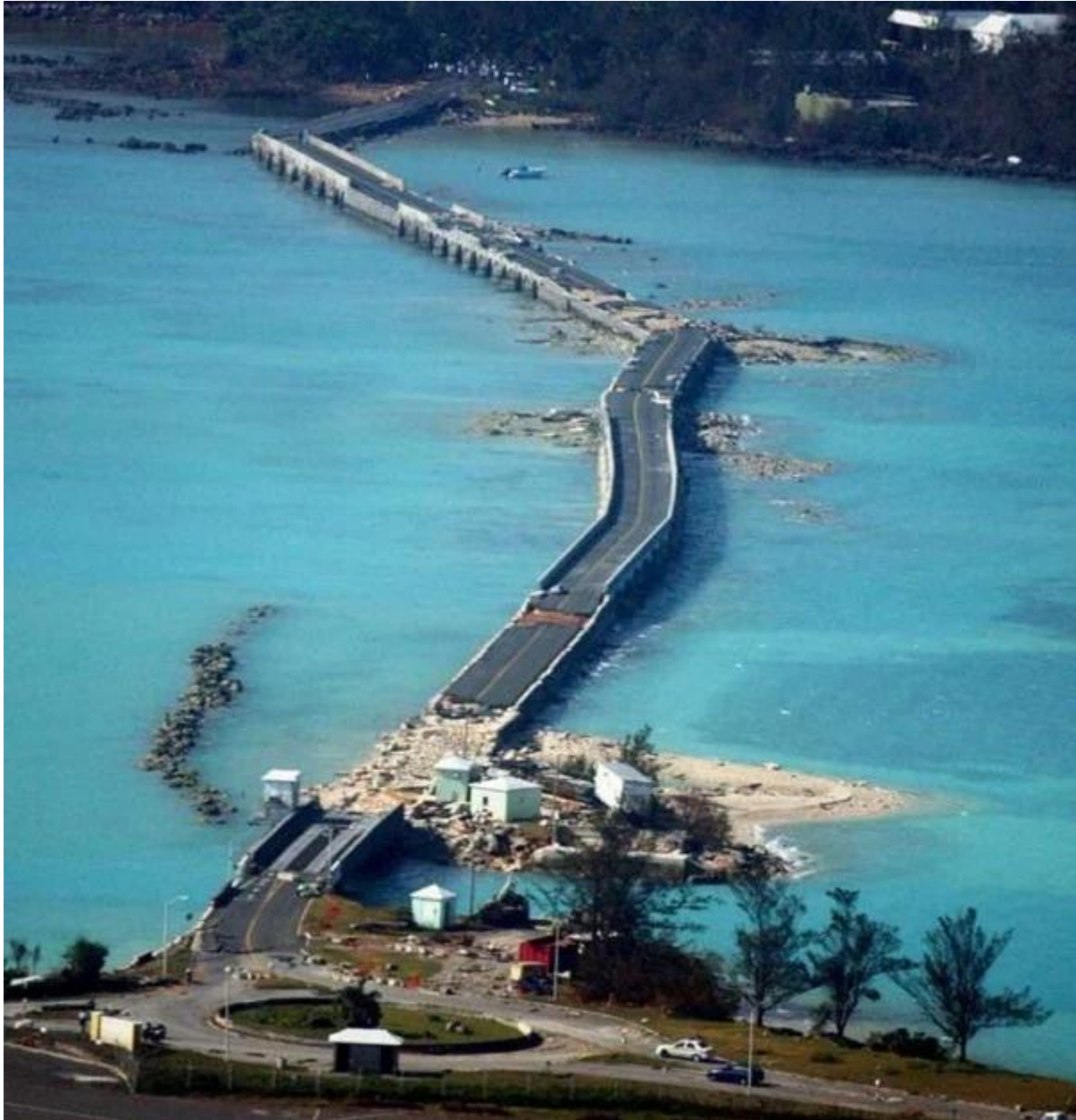
The Causeway, damaged by Hurricane Fabian, Sep 2003. ( www.royalgazette.com )
